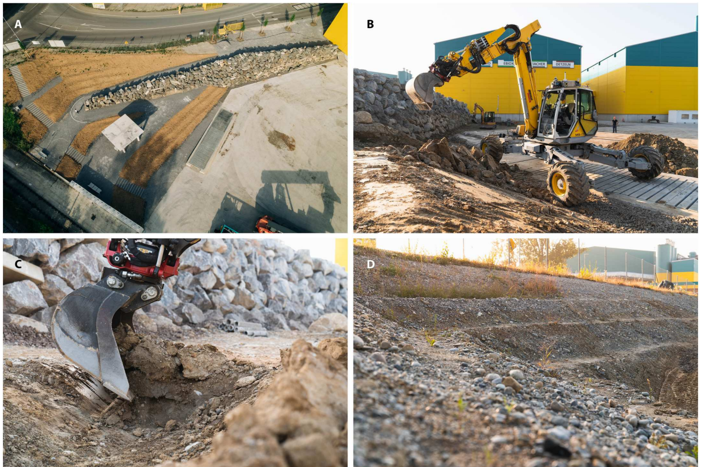
Fig. 5. Robotic landscaping. (A) Overview of park with integrated robotic terracing and stone retaining wall. (B) HEAP positioning to modify the lower slope with a grading bucket. (C) Grading bucket exit path while cutting the middle slope. (D) Intermediate berms on the sloped landscape for erosion control, displaying first signs of ruderal plant growth.
