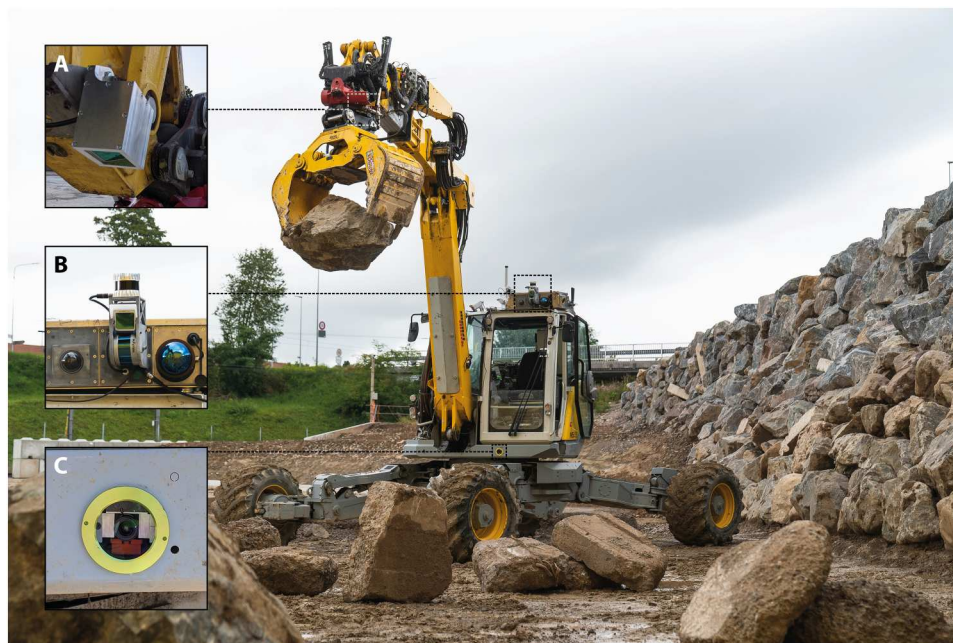
Fig. 1. HEAP is an autonomous excavator for construction with in situ resources. HEAP is a modified 12-ton walking excavator equipped with multiple cabin- and arm-mounted LiDAR sensors and cameras, facilitating the construction of the pictured 65-m-long retaining wall and terraced landscape from unmodified local materials. (A) Arm-mounted Livox Mid-70 sensor, (B) rooftop perception box with multiple LiDAR sensors and camera, and (C) lower-cabin camera.
