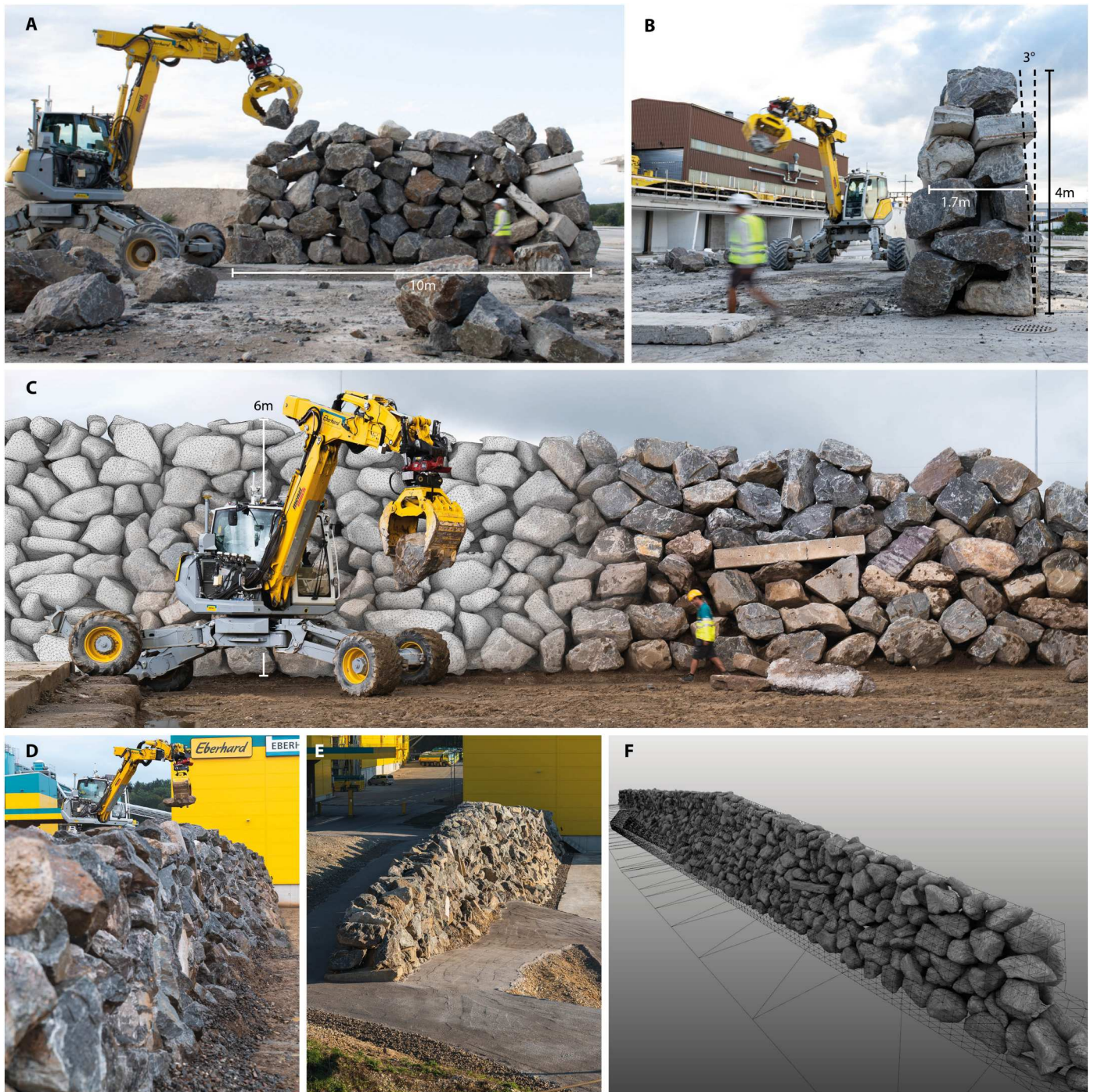
Fig. 3. Robotically constructed stone walls. (A and B) A 10 m-by-1.7 m-by-4 m freestanding wall built with 109 automatically digitized stones and reclaimed concrete elements. (C to F) A 65.5 m-by-1.8 m-by-6 m retaining wall built to comply with global geometric constraints. (C) Front elevation of retaining wall with partial overlay of mesh models from digital twin. (D and E) Overview of the built structure with variable height and incline. (F) Iteratively refined 3D digital twin model displayed in the geometric planning software.
